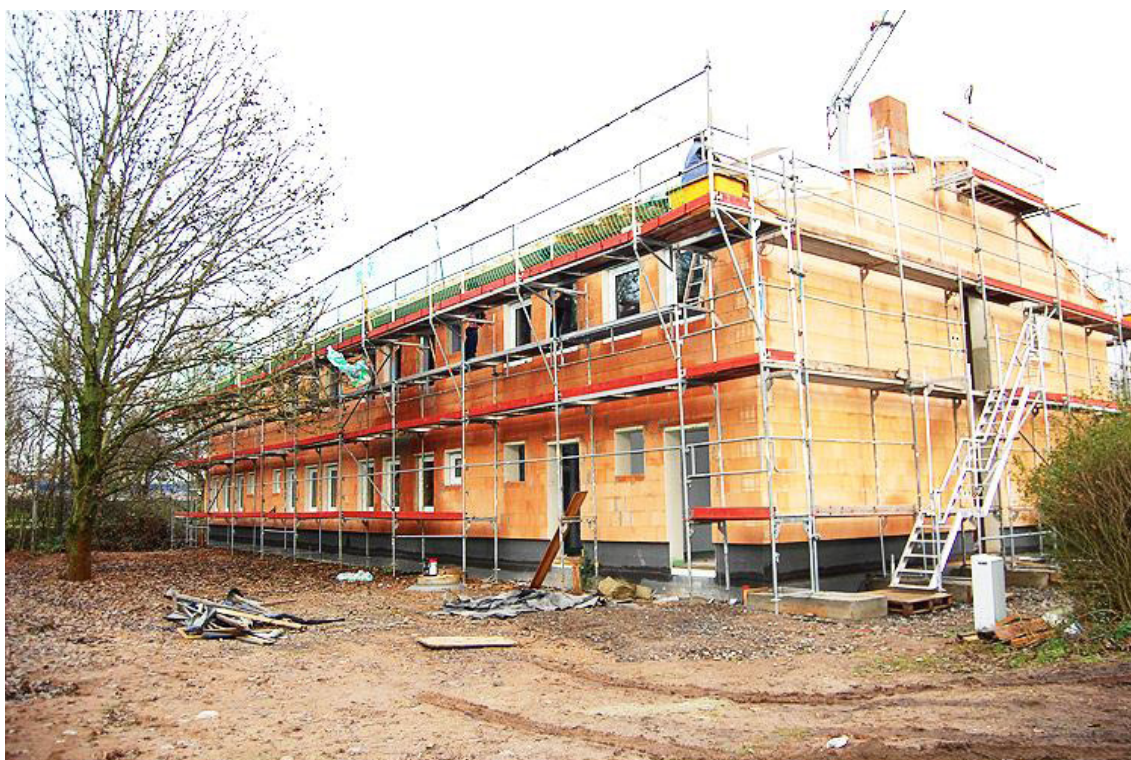
Figure 3. Construction of a refugee home, later used as a clubhouse and boarding school. © Sports club Budokan Maintal e.V.
